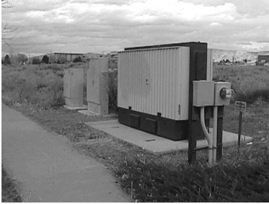
Figure 2 Avaya 80D Bulk Power DLC Telephony Cabinet
