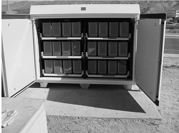
Figure 6 Batteries Inside a CoolCell™
