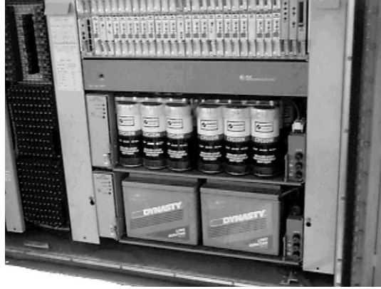
Figure 3 Batteries inside a Distributed Power 80D Cabinet
