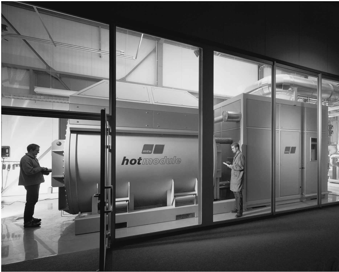
Figure 3: “View of the HotModule and CH 4 Humidifier and Heater”
