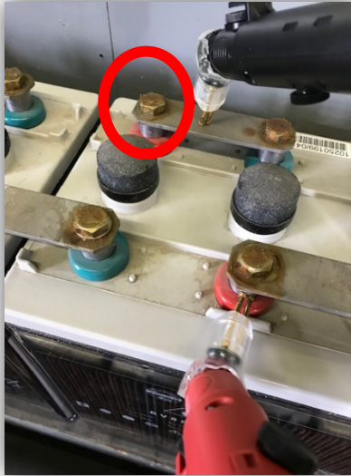
Figure 5. The intercell connection point NOT tested
