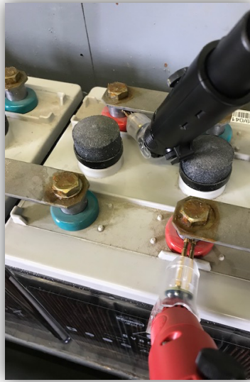
Figure 3. An intercell connection test
