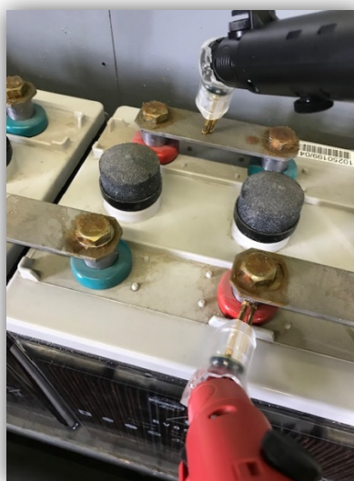
Figure 4. The incorrect intercell connection test
