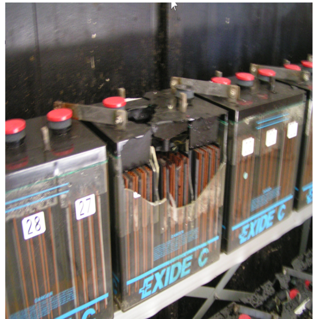
Figure 4. Explosion, damage propagated across the 3 cells, electrolyte still in these cells, low levels in other cells, part of cover and center vent missing, explosion originated in head space, damage limited to upper portion of cells, notice violence of event
