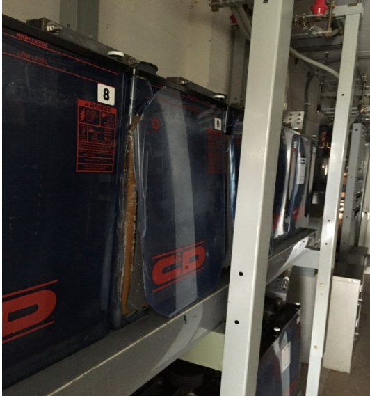
Figure 1. Ruptured cell caused by electrolyte freezing, bottom pushed out, side still connected to the cover, no violence displayed, parts pretty much intact but separated
