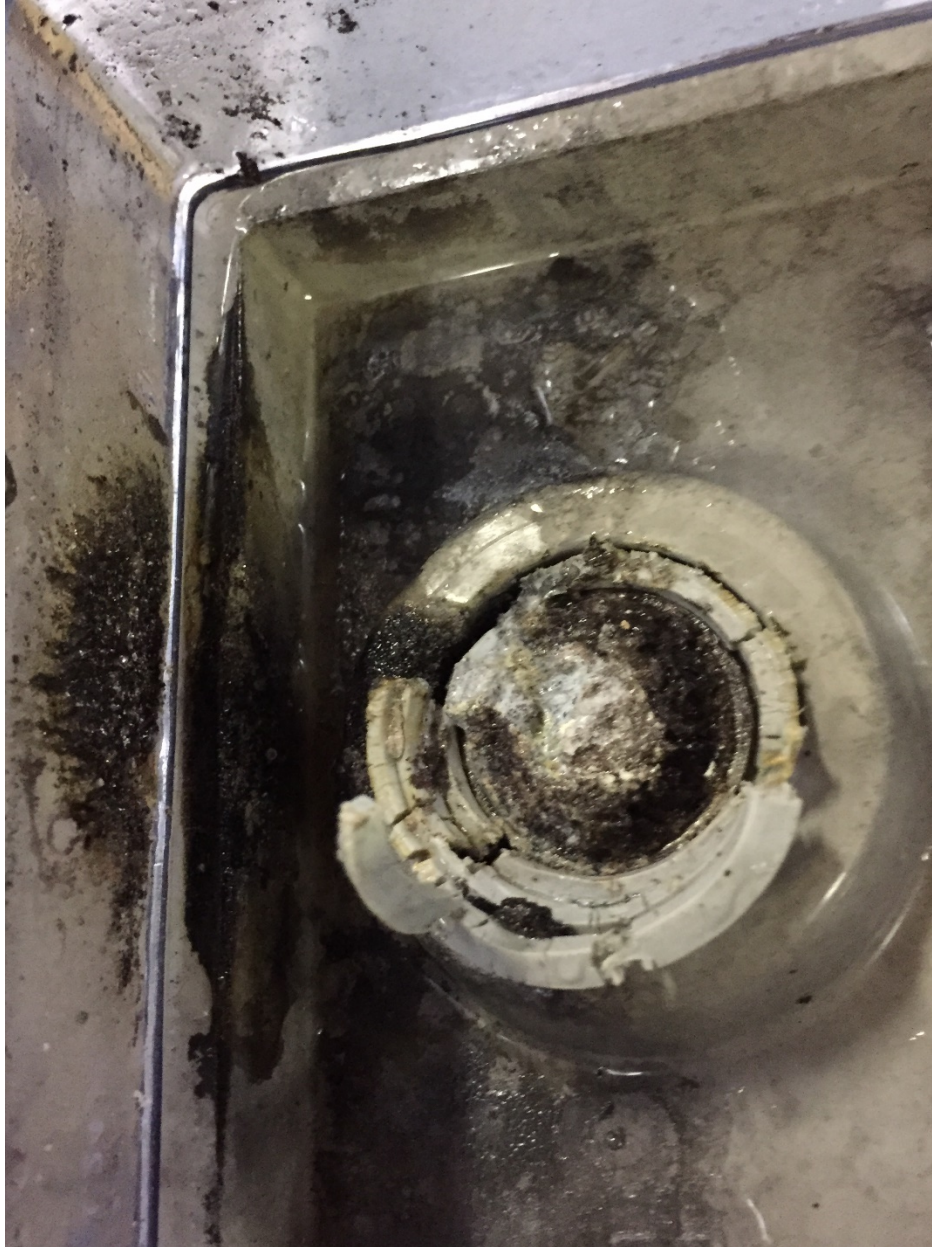
Figure 9. This positive post melted apart under load during first seconds of the unit trip. Notice metal splatter marks on bottom of this cover and side of jar. This cell DID NOT explode, because the mixture of gasses in the head space was not of the right combination that an ignition source could ignite it. The root cause failure investigation determined that nodular corrosion that had gone undetected during battery inspections was the cause of this battery failure. This battery had passed a recent discharge test, but because the discharge test was of a longer duration and lower current and did not include the inrush currents that would be required of the battery to support those instantaneous loads, this was not detected. If a modified performance test had been performed this would have been discovered during a planned outage instead of when the plant was operating. The generator required a rebuild, which as all involved in the utility industry understand, equals big $$$$ repair costs, plus the lost revenue while the rebuild is being performed. Not a good day for the home team.
