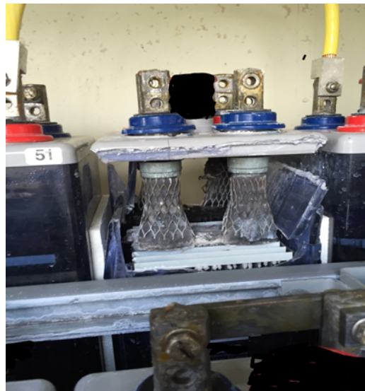
Figure 8. Explosion occurred during discharge test, nodular corrosion which is visible on the right rear positive post caused that post to open which created the arc that ignited the gas, as always with all cell explosions the damage is limited to the upper area of the cell, violent action
