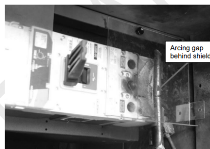
Figure 3-3: Test Fixture Mounted on Source Side of Circuit Breaker, with Shield
