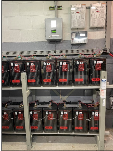
Figure 3. New monitoring device, pictured over cells 3 and 4, is installed in Dominion Substation
