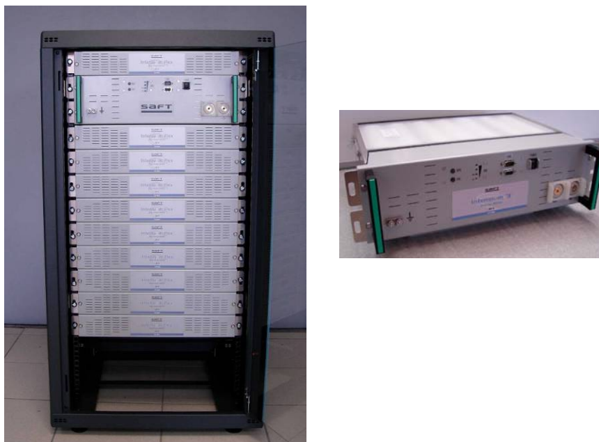
Figure 3 – 240 V and 48 V Modular Battery Systems
