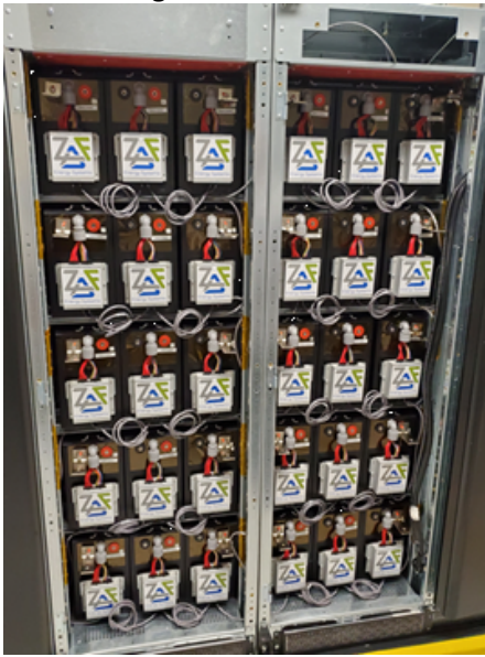
Figure 3: Data center cabinet containing Ni-Zn batteries (Courtesy of ZAF Energy Systems)
