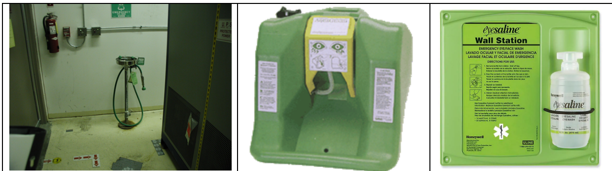
Figure 13 (Left) Note that flushing the plumbed eyewash station could spill water on the floor so people tend to neglect the requirement. Hence, this type of fixture rarely if ever gets flushed. (Right) Non-plumbed eyewash stations and bottles are easier to maintain.
