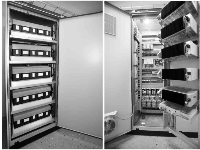
Figure 3. Left: each battery string is sitting on a sliding shelf, right: backside of chargers sitting on cabinet door plus five BMCs on left hand side wall.
